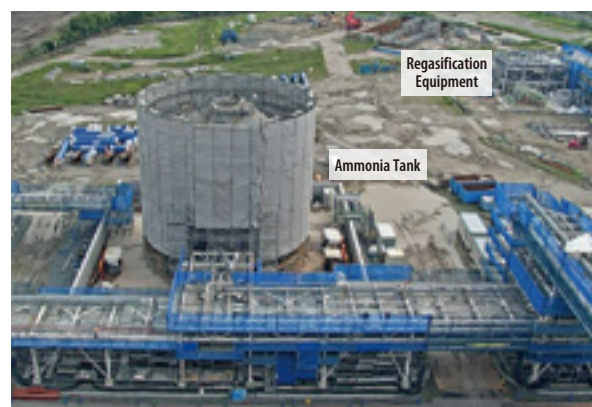
Construction Progressing on Ammonia Demonstration Test Facility at Hekinan Thermal Power Station
