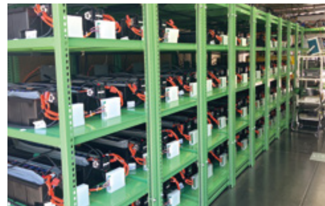
Large-capacity sweep energy storage system that uses electric car batteries
